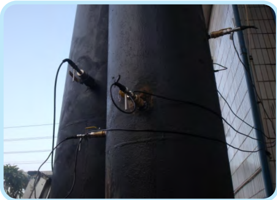
DN1000 Circulation Cooling Water
