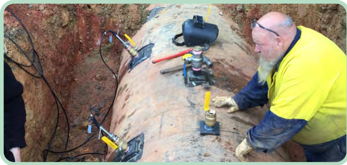
DN800 Water Supply
